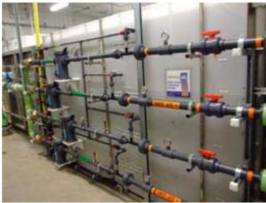
Ozonation Injection System
